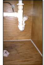
Monitor under a well-sealed sink
