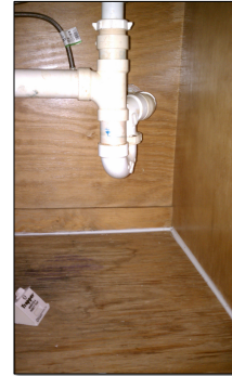
Monitor under a well-sealed sink
