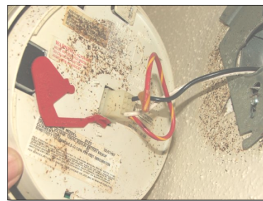
Cockroach infestation in a smoke detector
