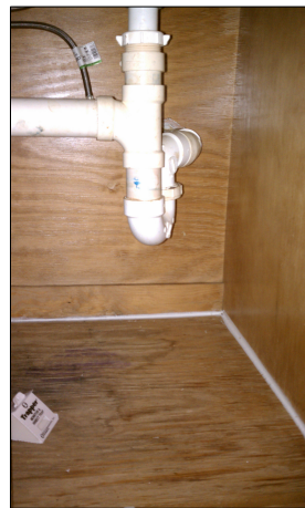
Monitor under a well-sealed sink
