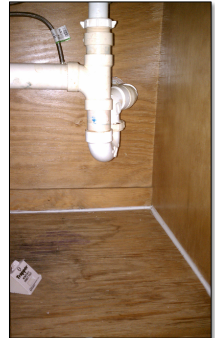
Monitor under a well-sealed sink
