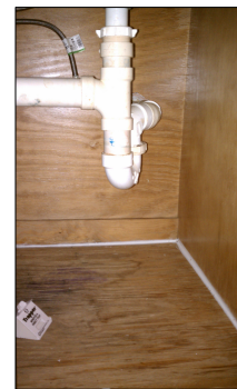
Monitor under a well-sealed sink
