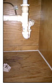
Monitor under a well-sealed sink
