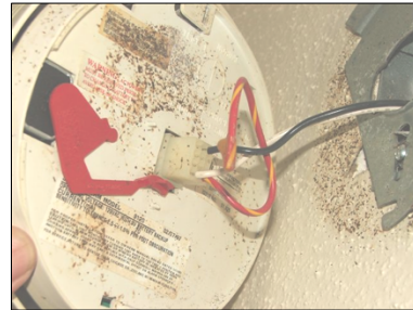
Cockroach infestation in a smoke detector
