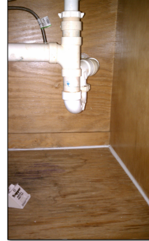
Monitor under a well-sealed sink
