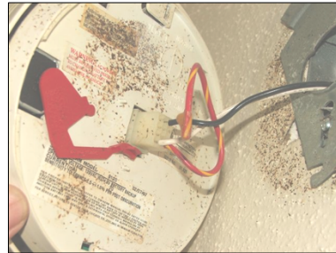
Cockroach infestation in a smoke detector
